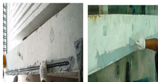
Figure 14. Post-collision application of steel jackets, polymer coatings, and FRP sheets on concrete girders and decks
