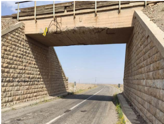
Figure 1. Railway bridge at kilometer 376+586 m subjected to over-height vehicle collision
