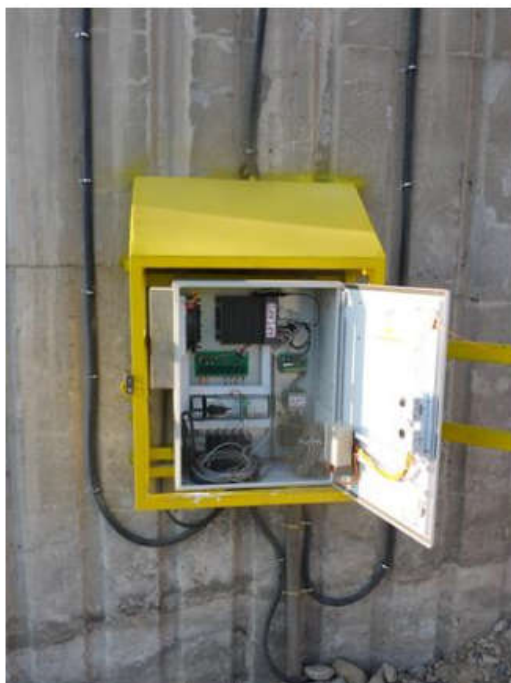
Figure 7. The central cabinet of the monitoring system
