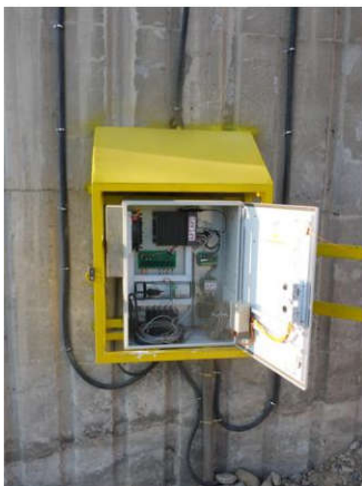
Figure 7. The central cabinet of the monitoring system
