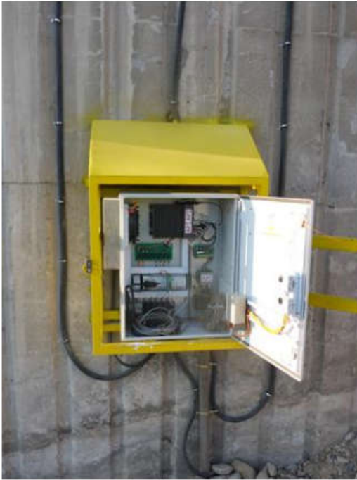
Figure 7. The central cabinet of the monitoring system
